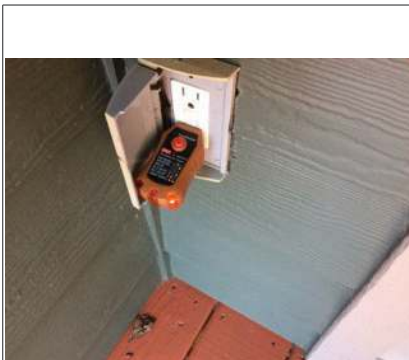
Exterior receptacle at back door is open neutral. Recommend consulting electrician for repair.
